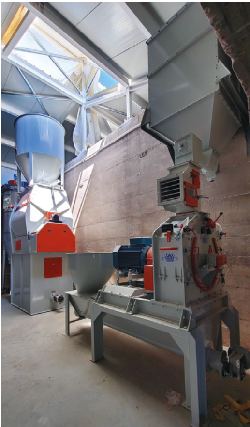
Briganti feed mill in Cortona, Ar, Italy. Plant for cleaning, storage and dosing of cereals and flours on 13 silos, total capacity 750 m 3 . Complete integration of the existing system with automatic cycles managed by the operator by means of PC and PLC.
