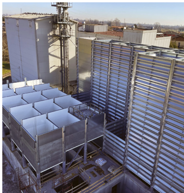
Complete storage plant under construction for Molino Cerere in Bassano del Grappa (Vi - Italy): batteries of prismatic corrugated cells for wheat and smooth cells for flour (Technobins).
